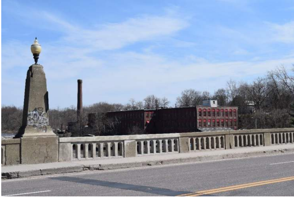
Photo 13: Bridge railing and ornamental details. Chace Mill in the background. Map ID 9.
