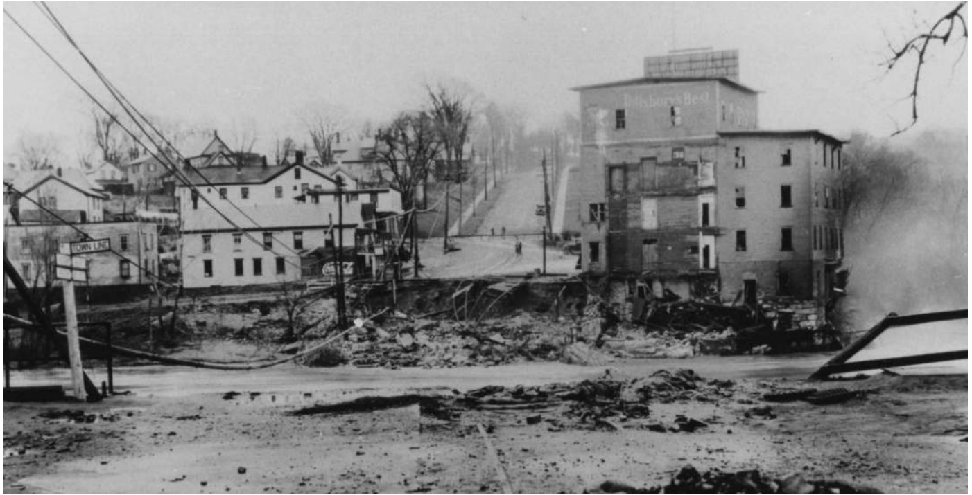
Figure 6: The Burlington Flouring Mill in the aftermath of the November 4, 1927, flood. The floodwaters severely damaged the building along with much of downtown Winooski and the OEE. To the left, Mill Street in the OEE is visible. 17
