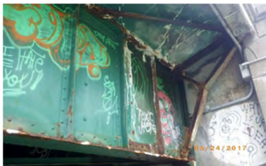
Fig. 5 – Typical Deterioration of Sidewalk Supports
