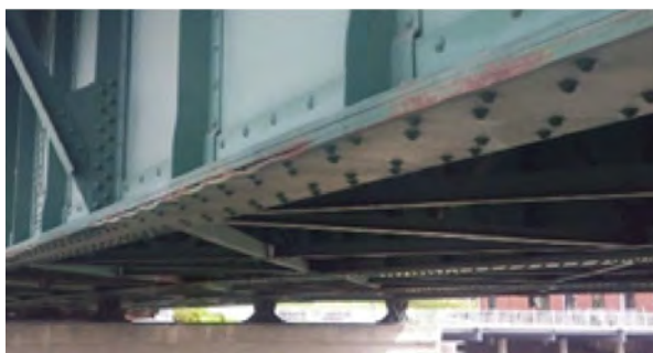
Fig. 2 - Typical Pack Rust Build-Up and Warping in Girder Bottom Flange
