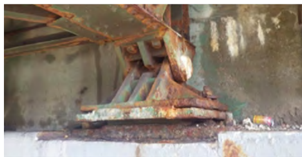
Fig. 3 – Typical Deterioration of Bridge Seats, Bearings, and Beam Ends
